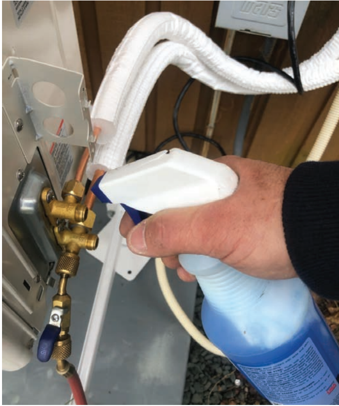
While the line sets are filled with high-pressure nitrogen, apply a leak-testing solution to all flares.
